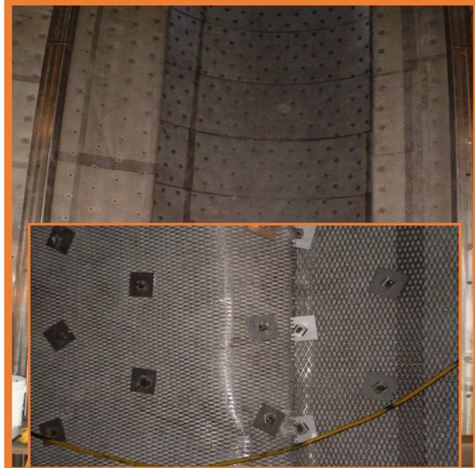
WRONG - Expanded Metal Liner Wire Welded Retainers
