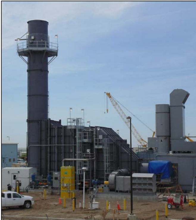
Basin Electric – LM6000 PC
